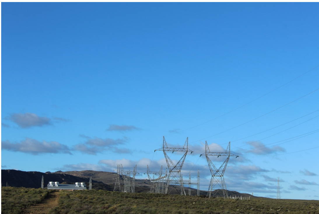
View of Quarry Traction Sub station
