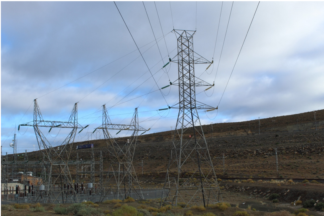
View of Laingsburg Sub station
