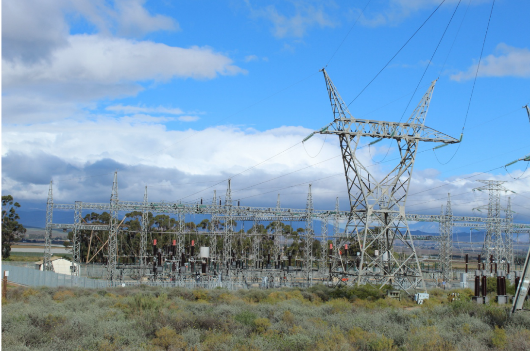
View of Boskloof Sub Station
