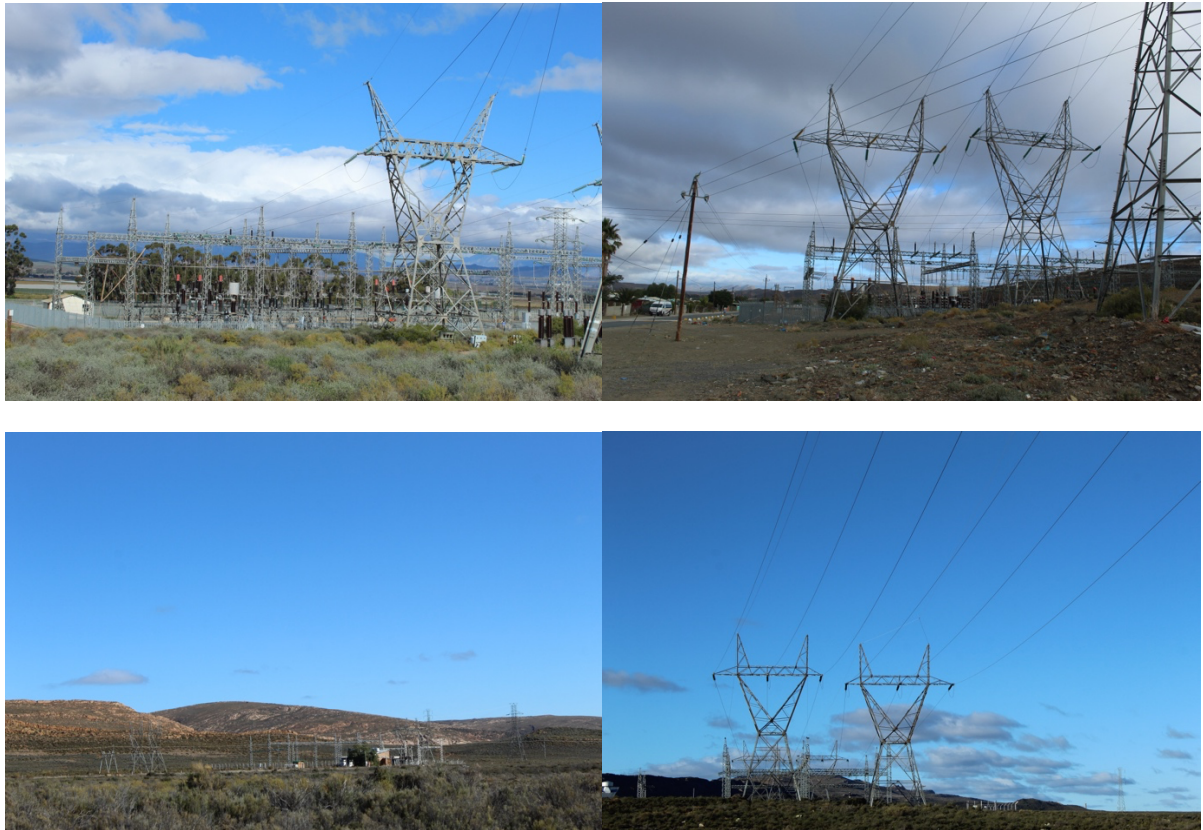
Figure 2: Picture of the Sub stations
