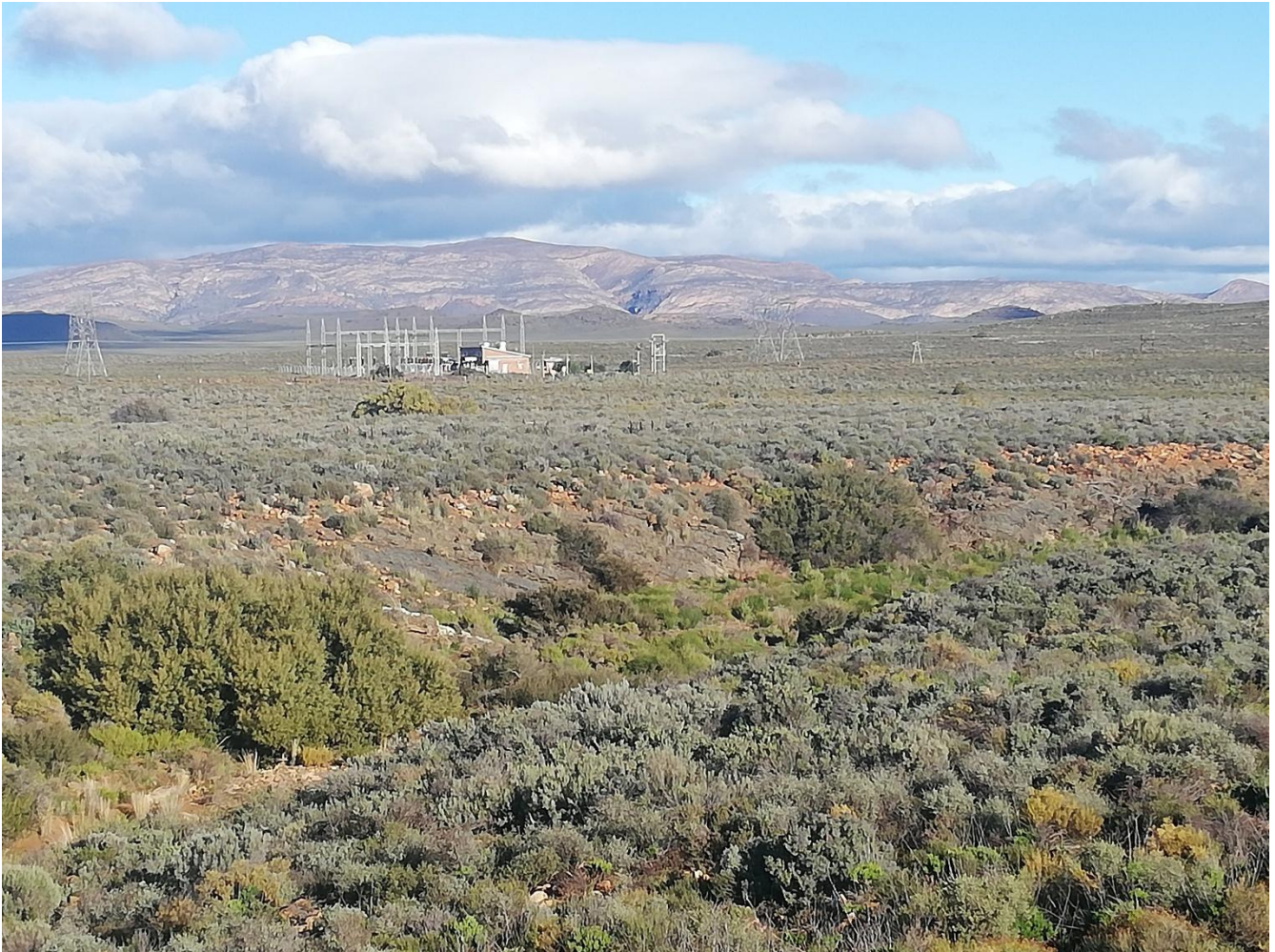
Figure 3: Photograph of a Substation taken during this report assessment powerline route site ground-truth site investigation (i.e. "Pietermeinties Traction Substation" along the Baviaans-Buffels River Catchment Watercourses). Note that the project area is located in a plain nested in a mesic natural succulent thicket ecosystem type.
