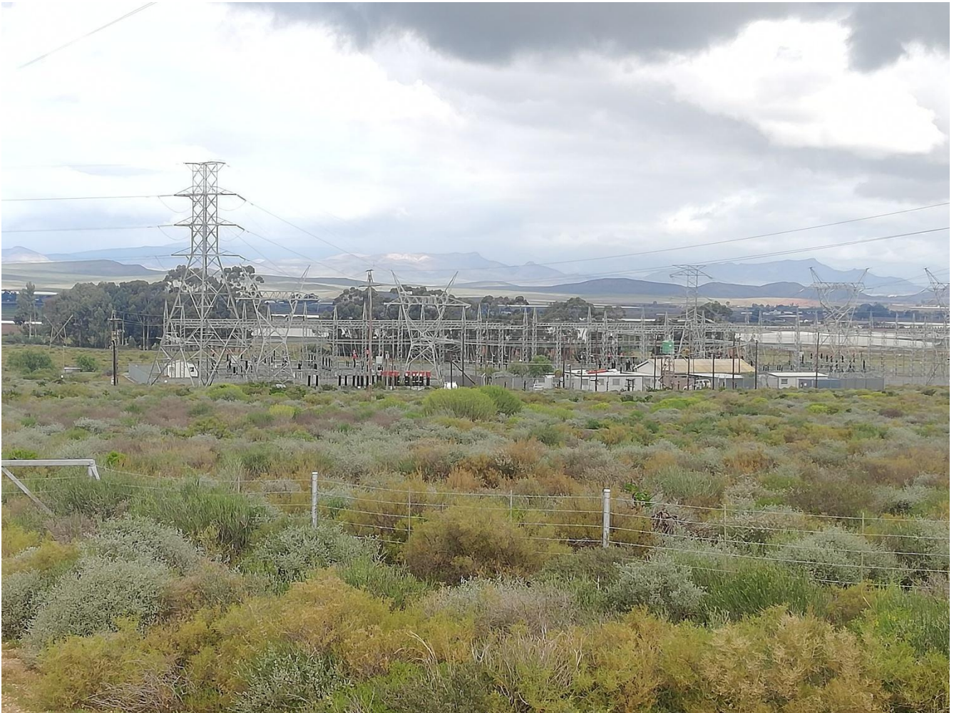
Figure 2: Photograph of Boskloof Substation taken during this report assessment ground-truth site investigation (i.e. affected Hex-Nonna-Nuy River Catchment Watercourses). Note that the project site is located on a mountain foothill and nested in a mesic natural fynbos ecosystem type.
