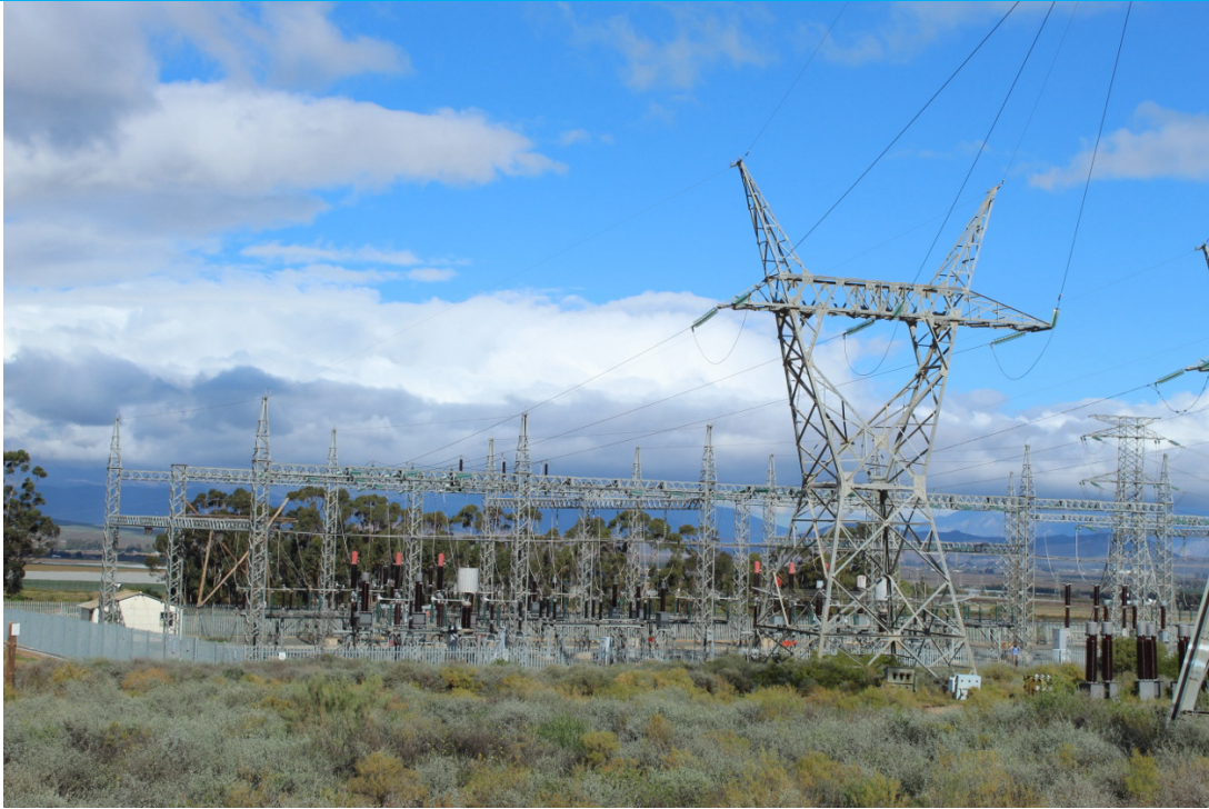
View of Boskloof Sub Station
