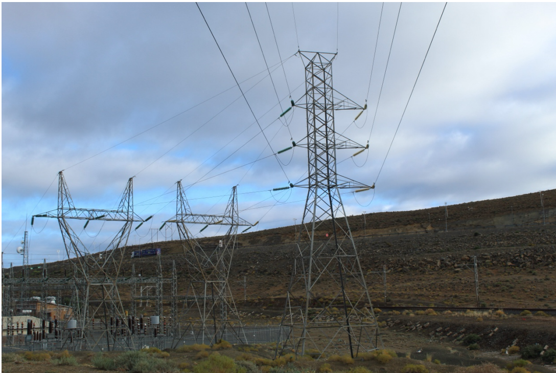
View of Laingsburg Sub station
