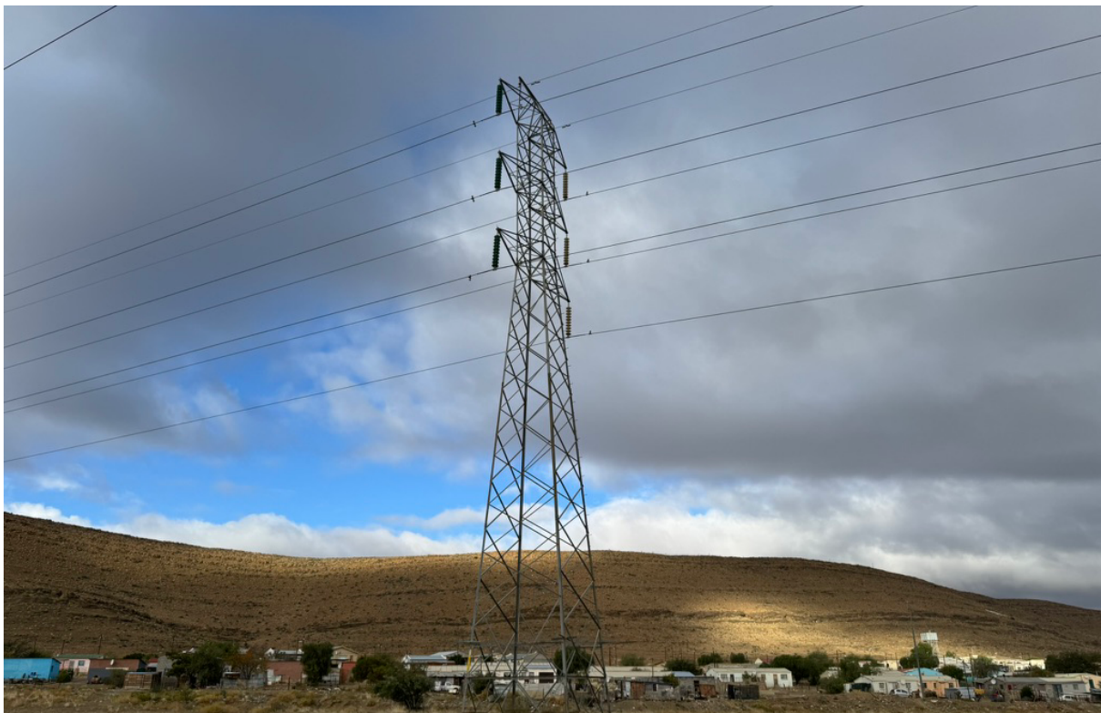
Figure 11: Lattice Tower Structure
