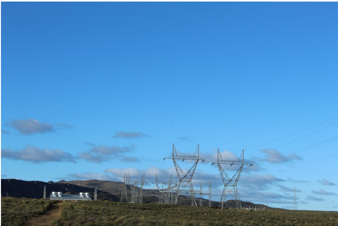
View of Quarry Traction Sub station
